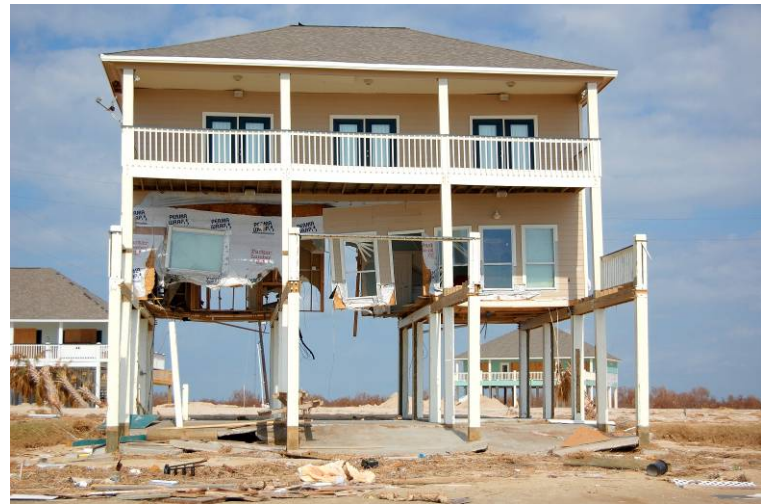
Figure 6: Newer construction in Biscayne subdivision in Crystal Beach, TX. Many beachfront homes sustained damage but homes set back from the beach exhibited minor damage.
