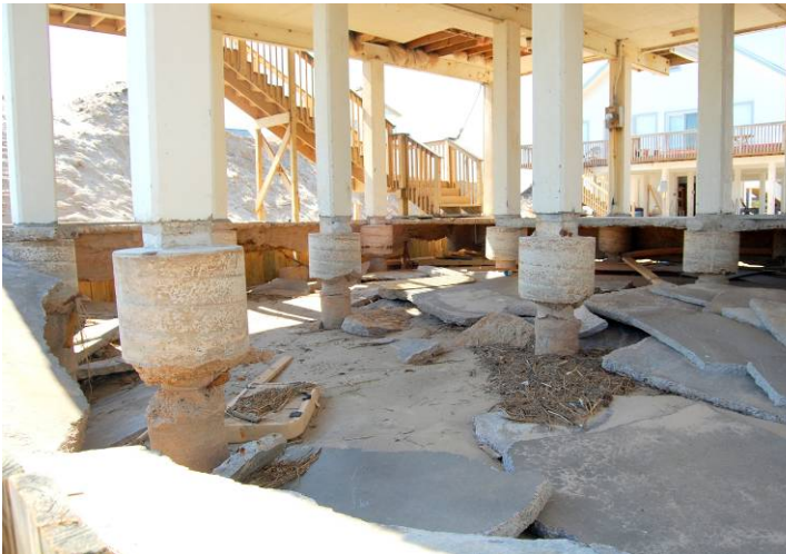
Figure 3: Typical slab foundation failure at beach-side residences
