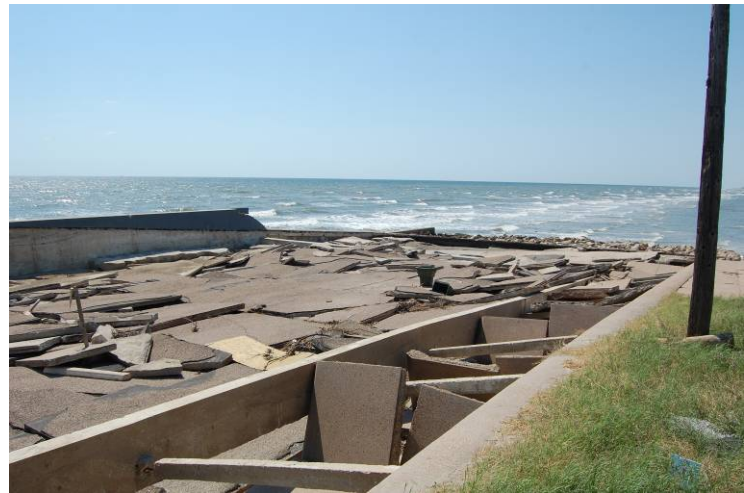
Figure 2: Road failure behind west end of seawall, Galveston, TX
